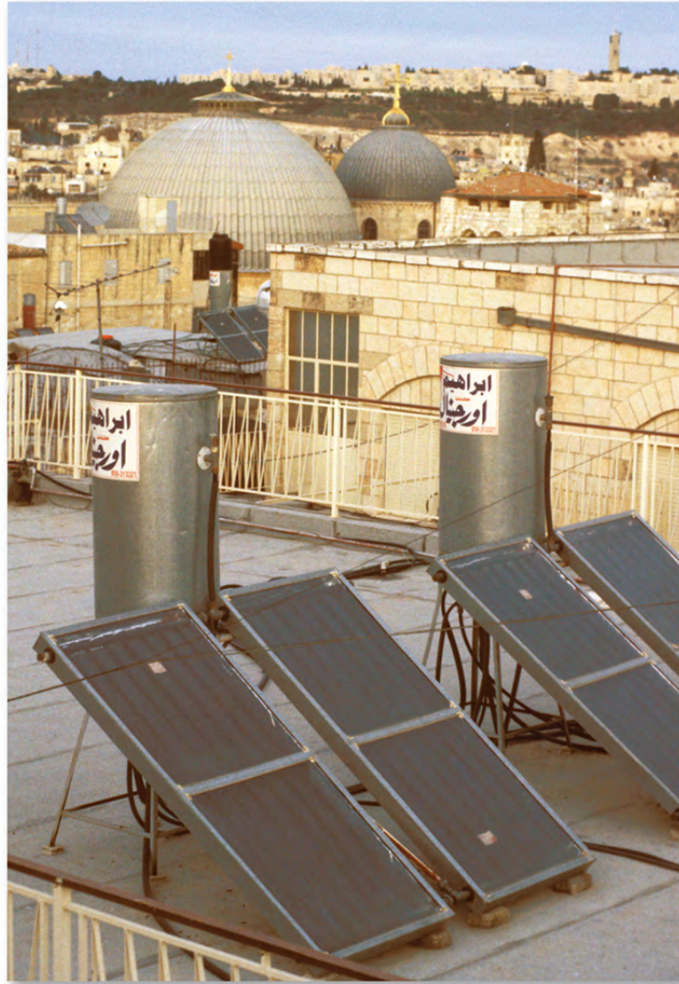
Figure 11-56: Solar energy heats water on this rooftop in Jerusalem.
